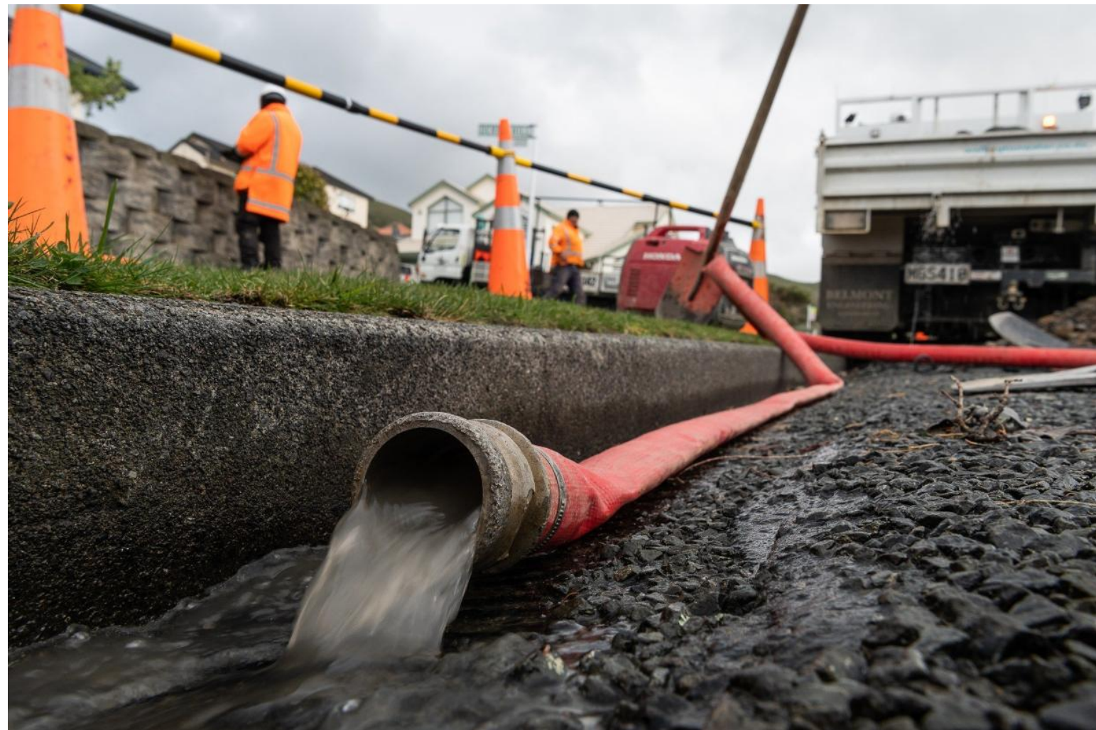
Fixing leaks is an expensive business for Wellington Water.
