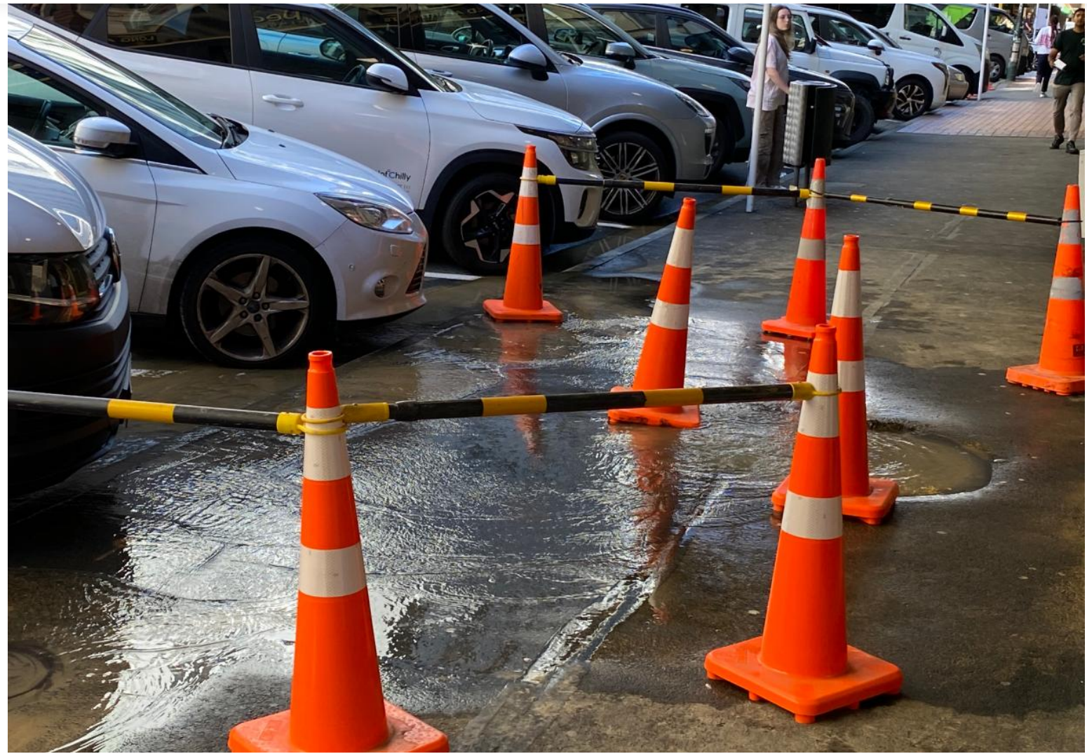
A water leak on Brandon St, Wellington, recently.
